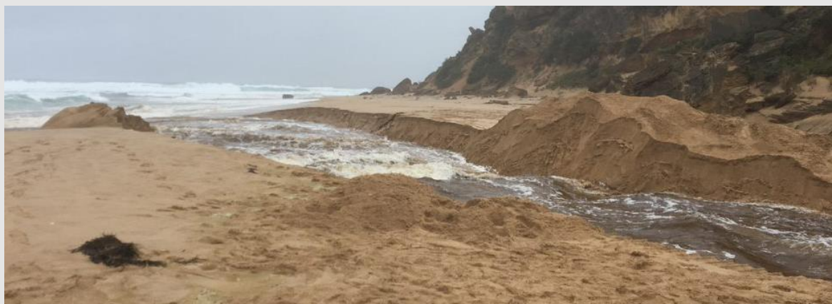
Photo: Excavation and artificial opening of the Aire River estuary on 23 May 2020. (Supplied: Parks Victoria)
