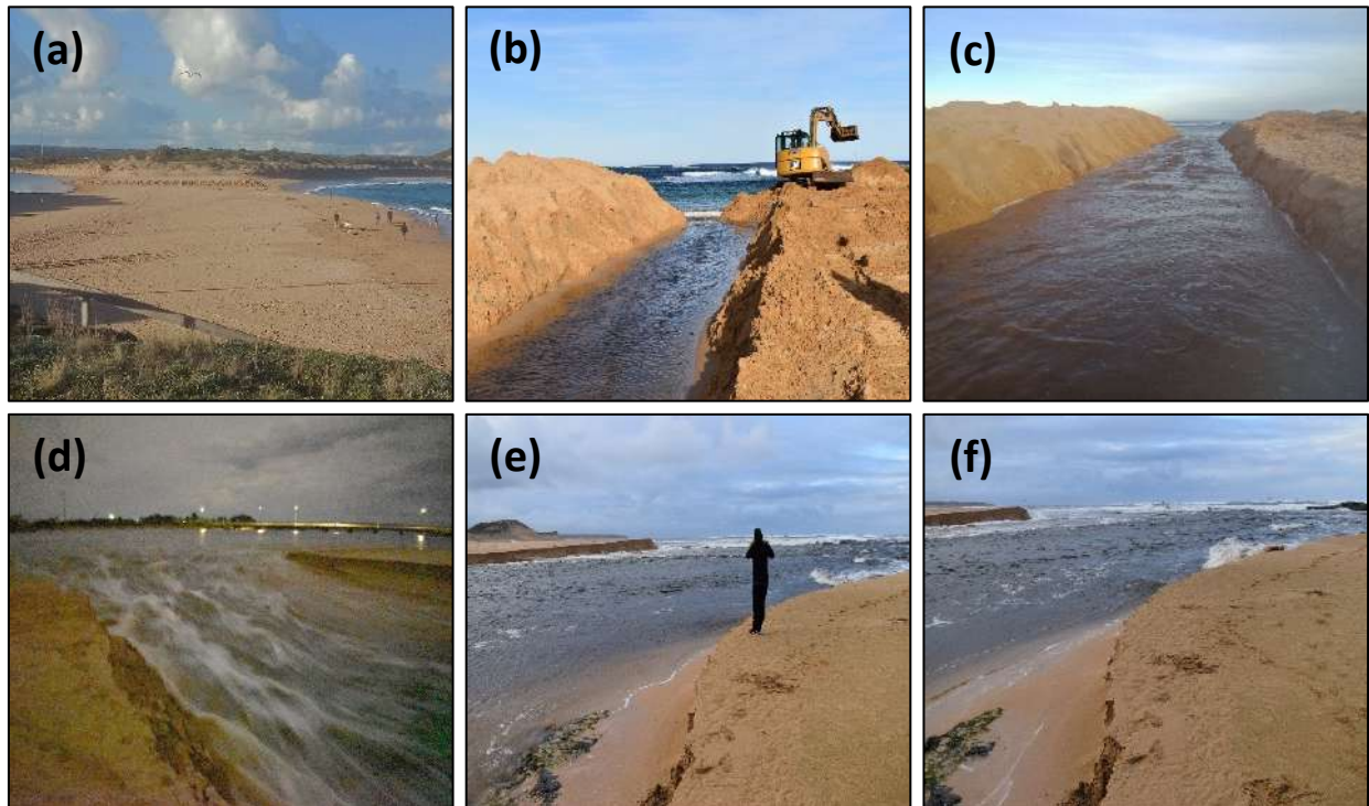
Figure 34a-f. Pictures from artificial opening 2 at Curdies Inlet. (a) 9 am 17/06/19 prior to opening; (b) 3 pm 17/06 excavation; (c) 5 pm 17/06 channel expansion; (d) 2.50 am 18/06 near peak outflow with standing waves (picture brightened); (e) 8 am 18/08 peak discharge; (f) 11 am 18/06 wave intrusion.
