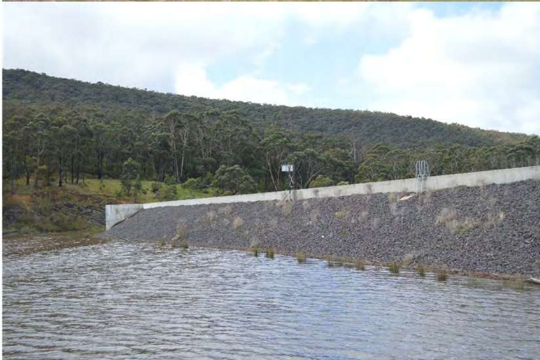
Figure 1.5 A) Downstream and B) upstream face of Painkalac Dam at full capacity (2017). Environmental flows are delivered by opening the valves within the fenced plumbing.
