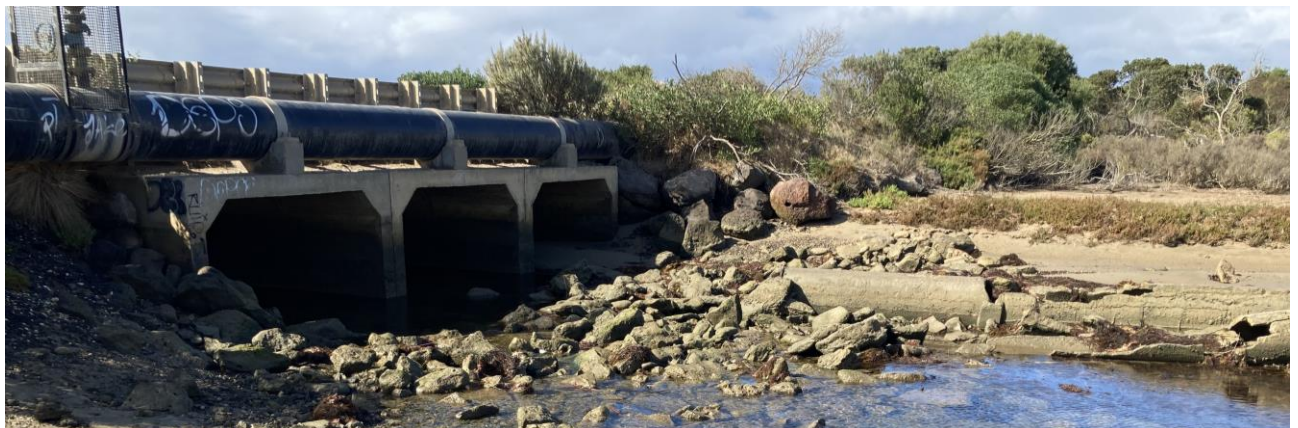
Figure 7 Photo of the culverts beneath Point Impossible Road connecting Mullet Creek to the Thompson Creek estuary
