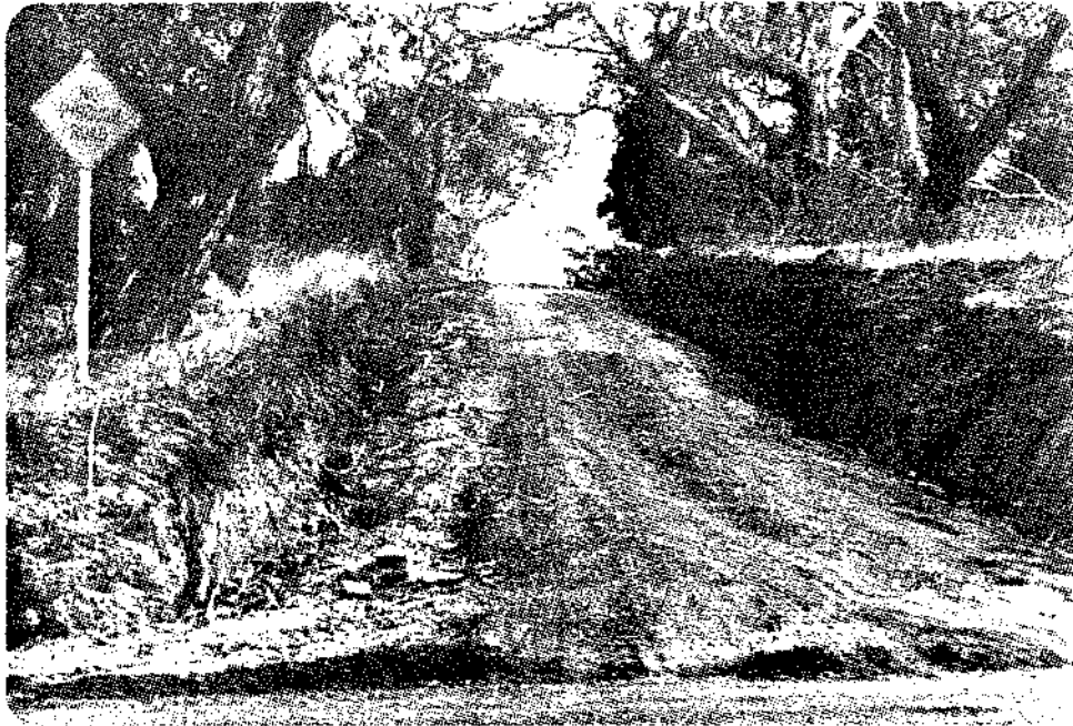
Photo 10 : Corner of Pearse Road and Aireys Street. A poorly constructed and surfaced road subject to severe erosion.
